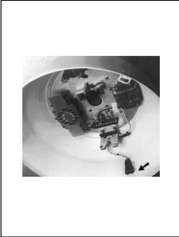
Figure 1. Back Box Power Switch Location
